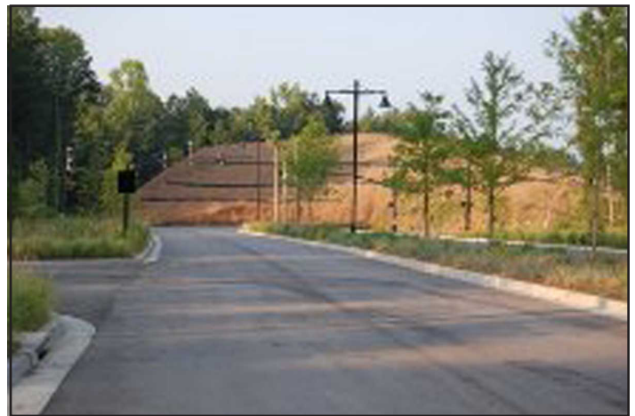
Figure 24: The image shows a section of roadway under construction on July 5, 2012. The roadway skirts Bluehouse Swamp and traces the original footpath to Woodstock Plantation. Image is courtesy of Ann Yarbrough.
